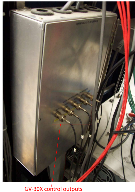
Figure A.22: Control Rack - rear breakout #2
