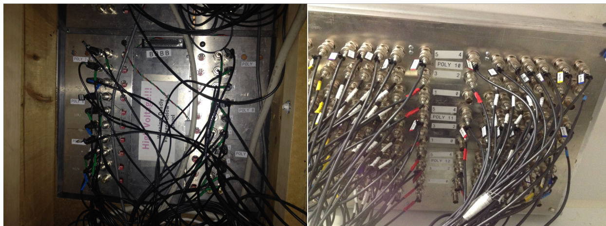
FIGURE 4.4: These pictures show the “feedthrough panel” in the Thomson detector/laser room before the upgrade. The feedthrough panel resided in the ceiling of the room/the floor of the mezzanine above the room. The photo of the left (A) is a view from the mezzanine and the photo on the right (B) is the view up from the laser room.
